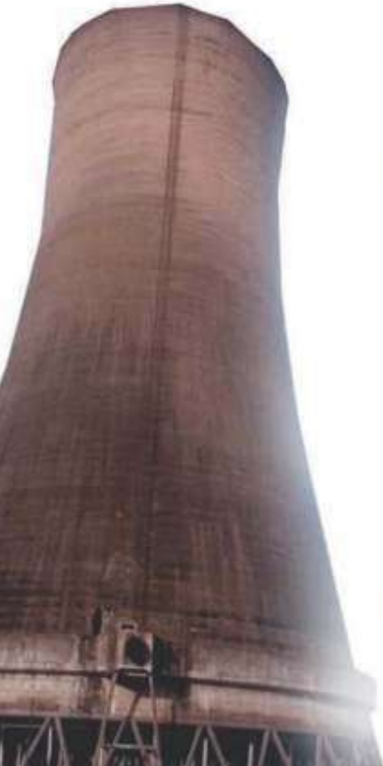
For the first time in India Demolition of Super Structure by CONTROLLED DEMOLITION
